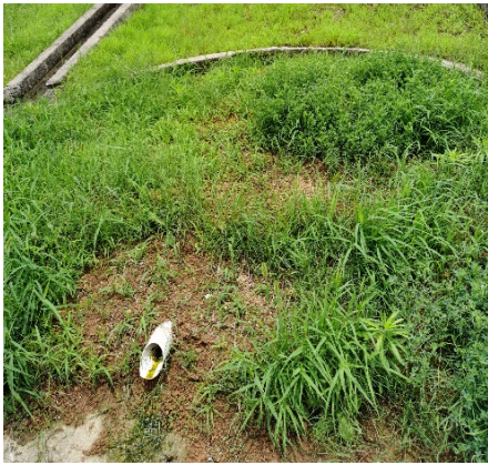
Fig. 17 Second slope in the 9+180
