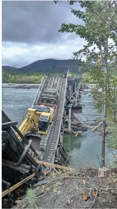
Figure 1. Bridge collapse over Minkule River, Siberia. August 2016. Photograph: Olga Ulturgasheva.
