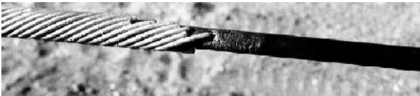
Figure 3. Damage on a polyethylene sheathed cable on a 110 kV line. The metallic wires on the left are part of the cable clamping system at the tower.
