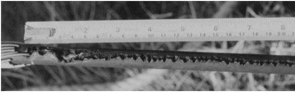
Figure 2. A photograph of cable damaged on a 400 kV line in the UK. The deep trough in the sheath is visible on the underside of the cable. The metallic wires on the left of the picture are part of the clamping system.
