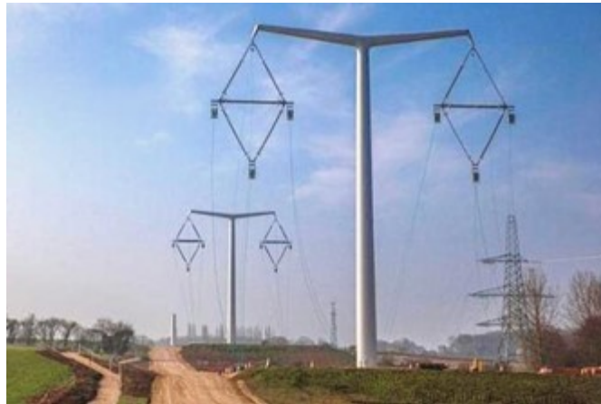
Figure 1. First T-Pylons erected as a trial in 2015 by Balfour Beatty at Eakring
