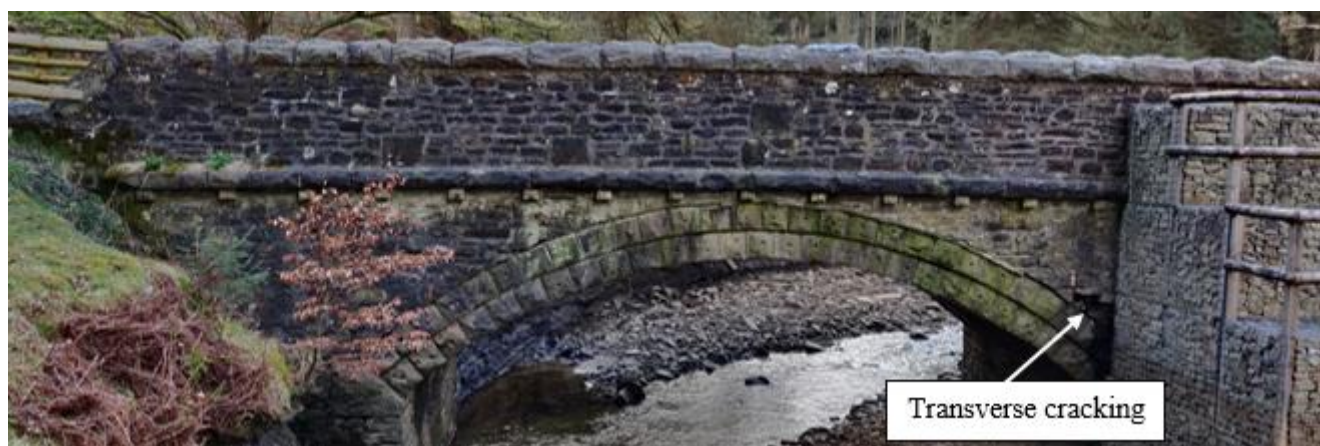
Figure 1: Downstream elevation of a single-span masonry arch bridge in Derwent Reservoir, Derbyshire, UK (image by Eda Majtan)
