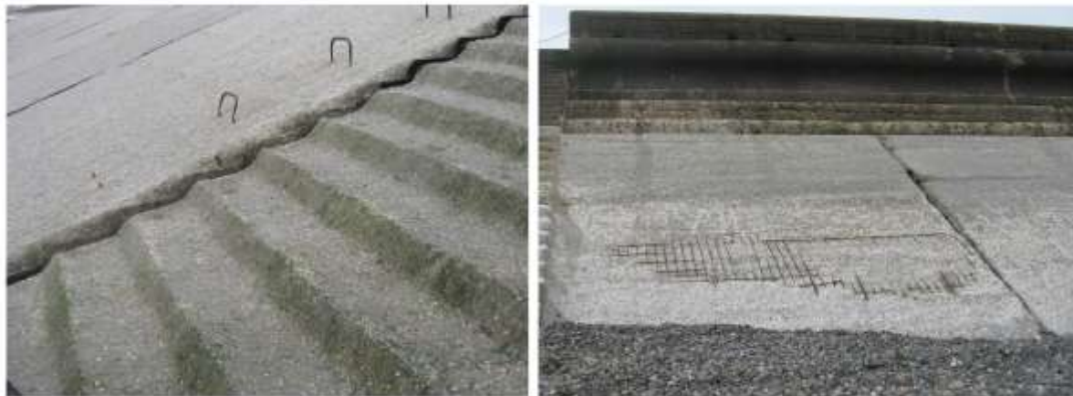
Figure 1: Abrasive wear at beach access steps (left) and sloping apron (right)
