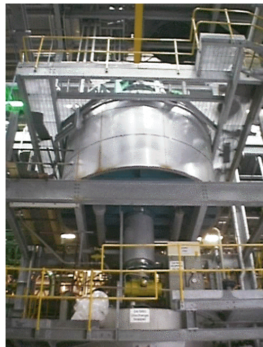
Figure 6.2: Underside view of filter 24/970
