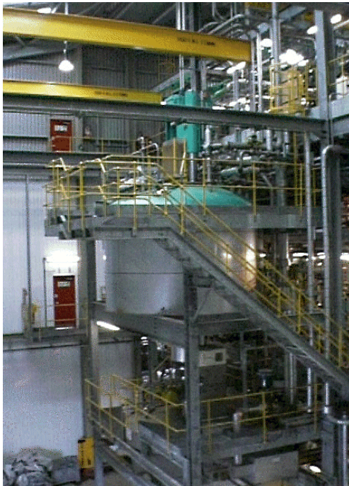
Figure 6.1: Side view of filter 24/970
