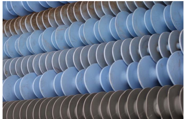
Figure 1. Insulators comprising the reference cross-arms
