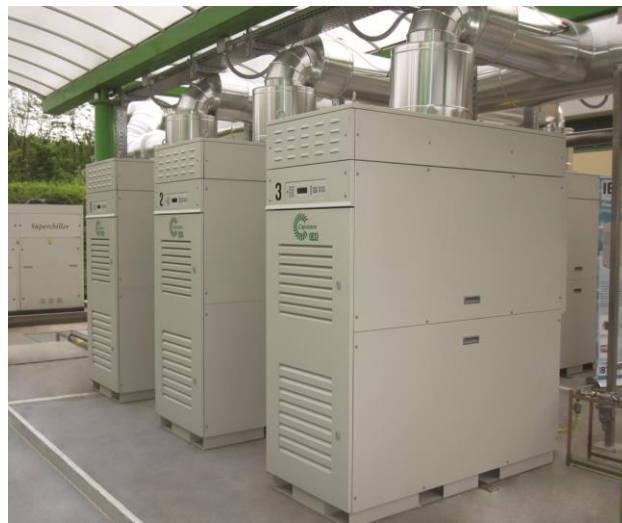
Figure 48 Set of micro-turbines (Picture provided by Capstone Turbine Corporation).
