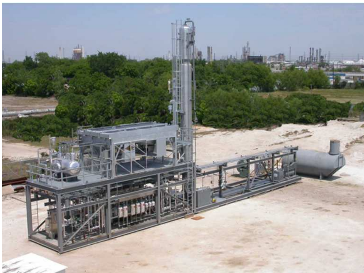
Figure 3: Modularized distillation system includes boiler, fractionator, overhead condenser, heat exchangers, pumps and controls. Photo used with permission from Mr. Bill Stanley.
