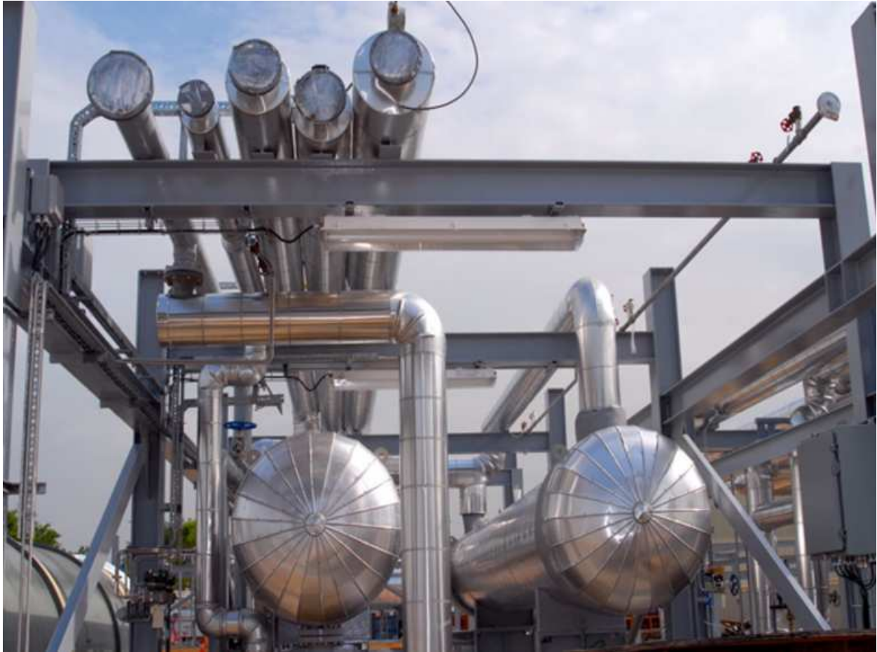
Figure 1: A shipping container-sized module consisting of two heat exchangers. The top of the module serves as a pipe rack. Photo used from permission from Mr. Bill Stanley.
