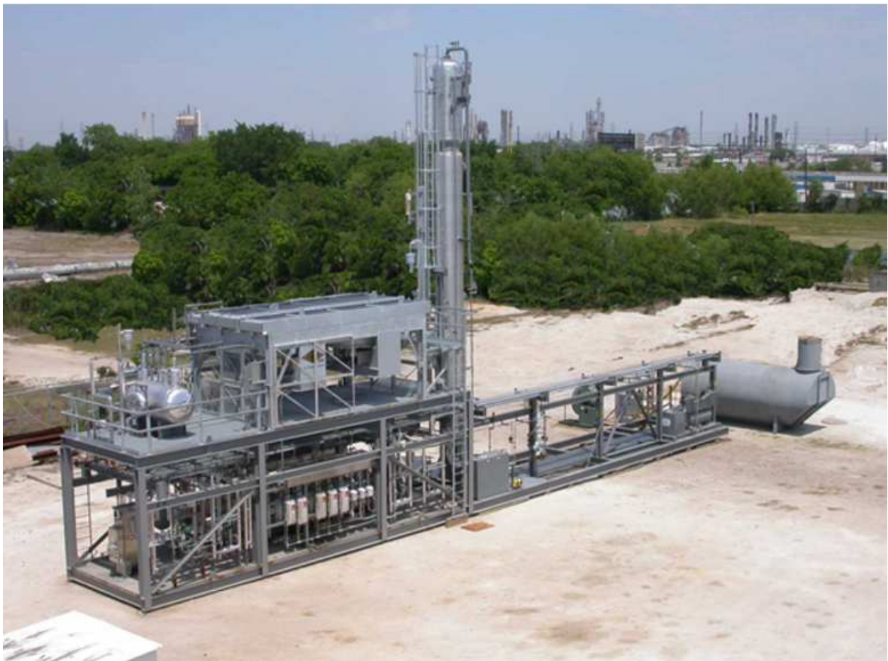
Figure 3: Modularized distillation system includes boiler, fractionator, overhead condenser, heat exchangers, pumps and controls. Photo used with permission from Mr. Bill Stanley.
